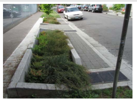
Bioretention planter in the landscape strip manages stormwater runoff in the ROW. See below for standard engineering plan for a similar facility. (Photo courtesy Muralmouth.Wordpress)
